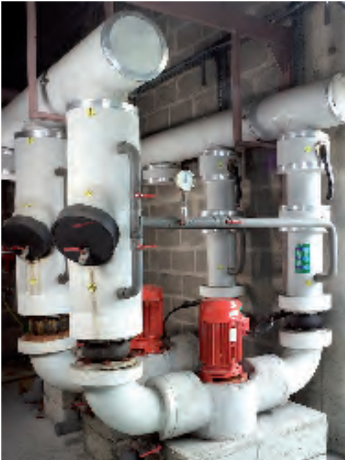
Example of pumping application using the Altistart 22 soft start - soft stop unit
